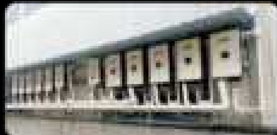
Product: Three-phase 20kW Project Size: 200kW
