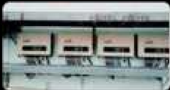
Product: Three-phase 60kW Project Size: 500kW
