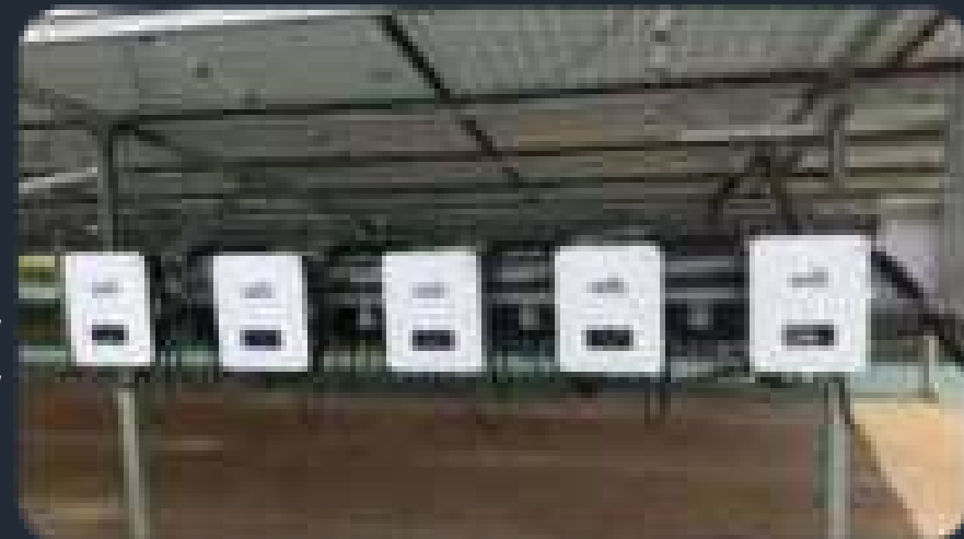
Country: Japan Product: Single-phase 5.5kW Project Size: 49.5kW
