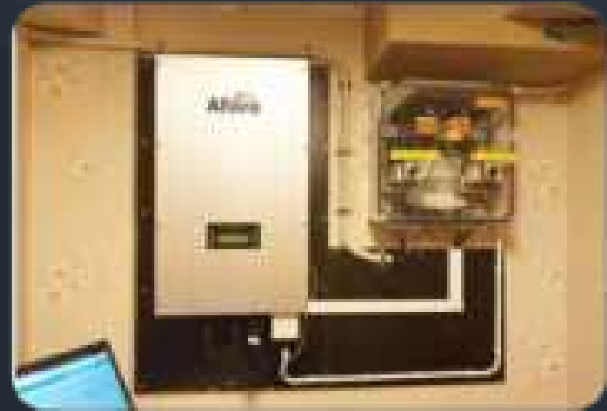
Country : Norway Product : Three-phase 15kW Project Size : 15kW
